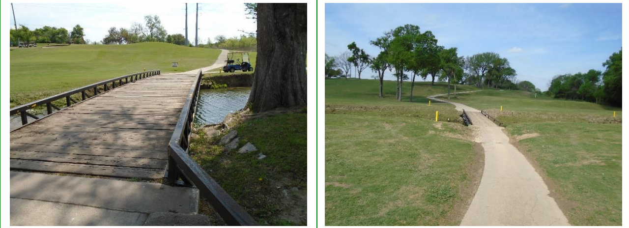
Photos showing the bridges on MWGC with wooden planks that tend to wear out and must be replaced every 10+/- years.
