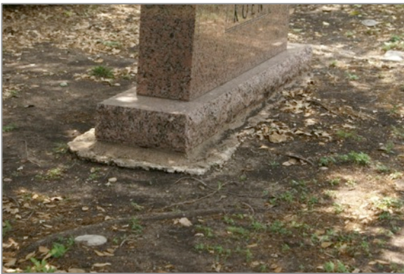
Visibly thin exposed foundation, Austin Memorial Park Cemetery, Section 2
