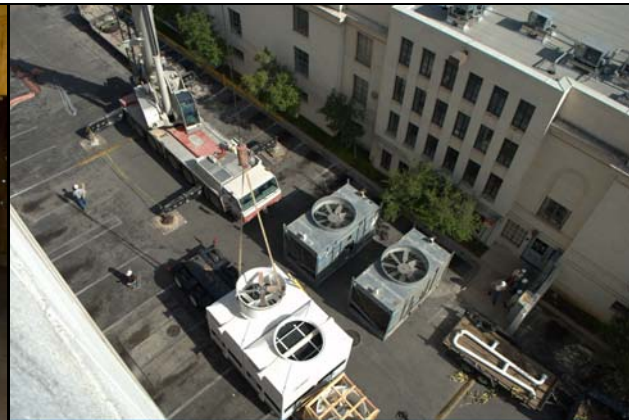
JHF/AHC Cooling Towers
