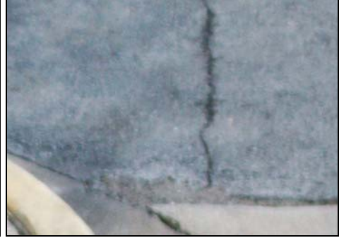
Sewer Line: Cracks in Parking Lot
