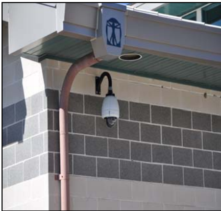
Exterior Security Cameras
