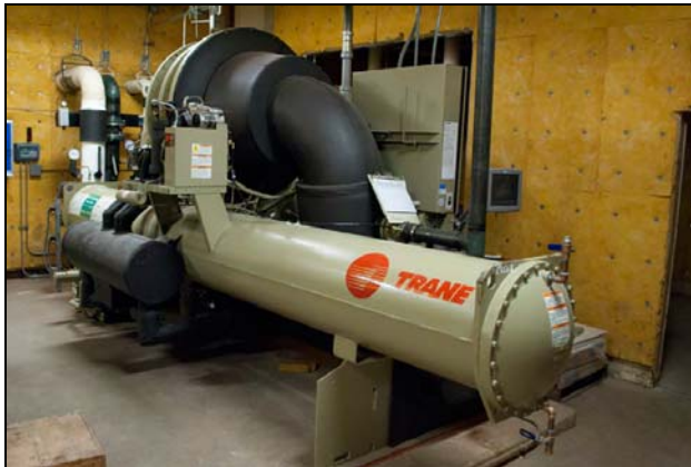
JHF / AHC Chiller
