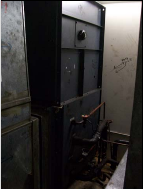
Pleasant Hill HVAC Unit
