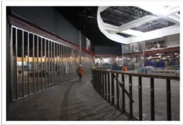
System Control Center
