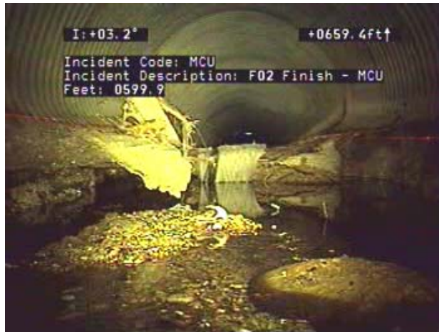
Damaged infrastructure in Hether St. storm drain system
