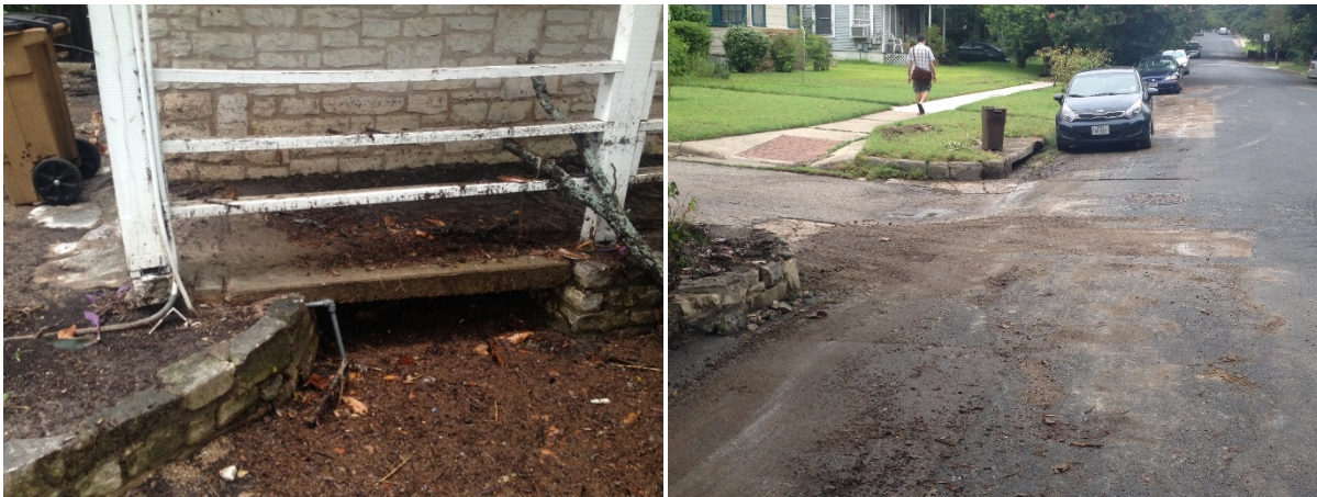
Localized flooding damage at 34 th Street and Fruth
