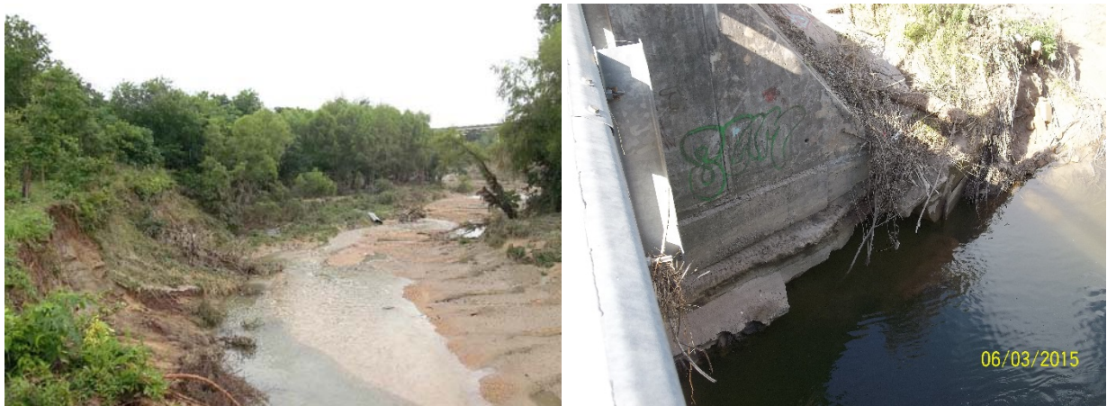
Channel erosion on Boggy Creek east of 183 threatens the Delwau Bridge
