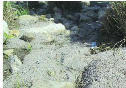
Sediment in Rain Garden
