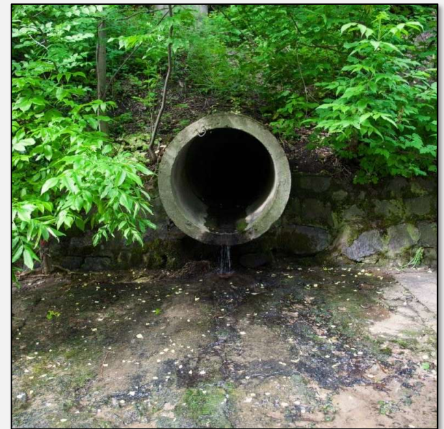
3. Rainwater is released into a creek at the outfall. Sometimes it goes to a water quality or detention pond first.
