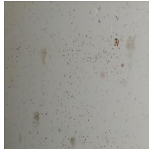
Water leaks = mold hazards
