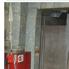
Broken ducts = higher heating bills
