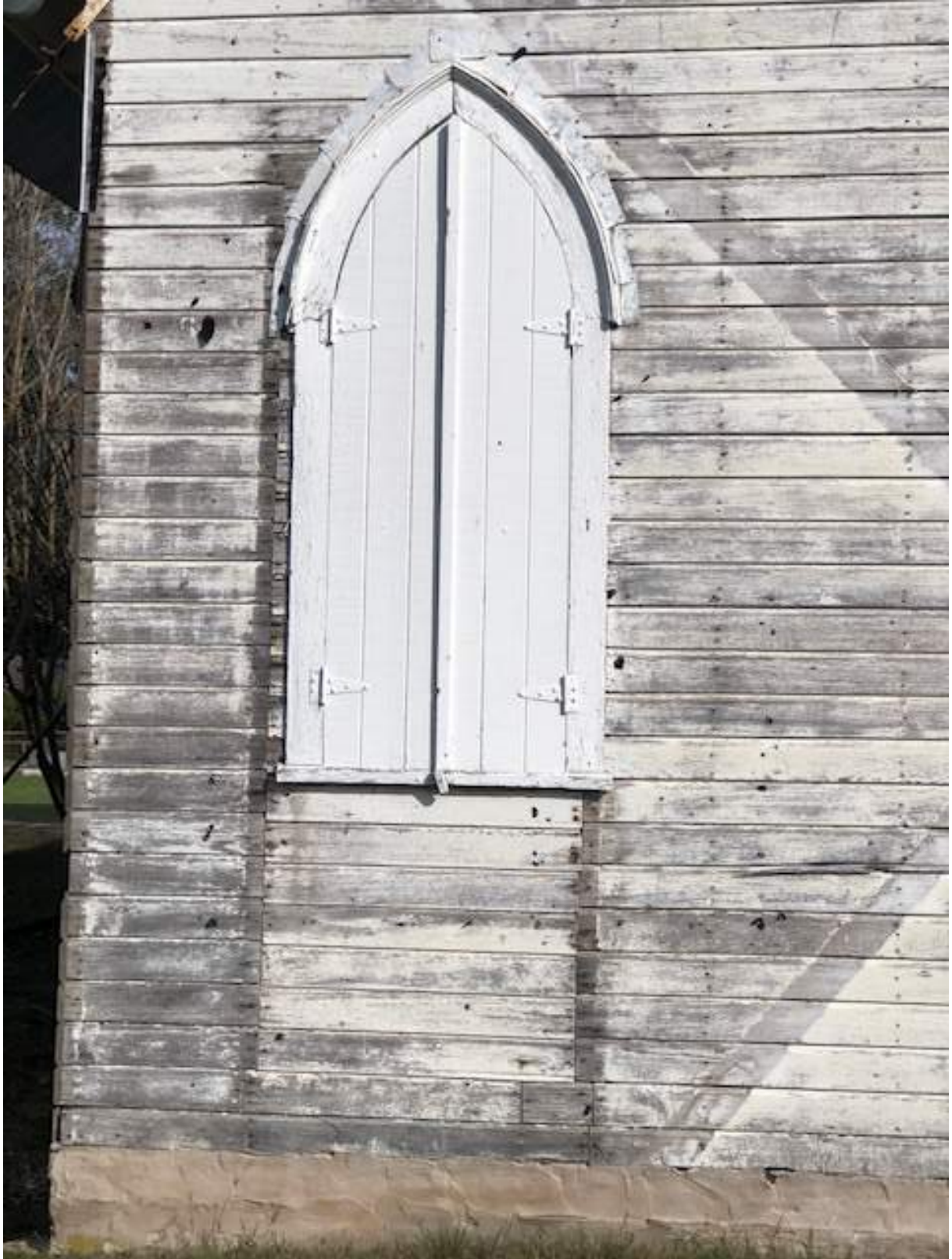
Detail of rear shows where window was moved to replace a back door.
