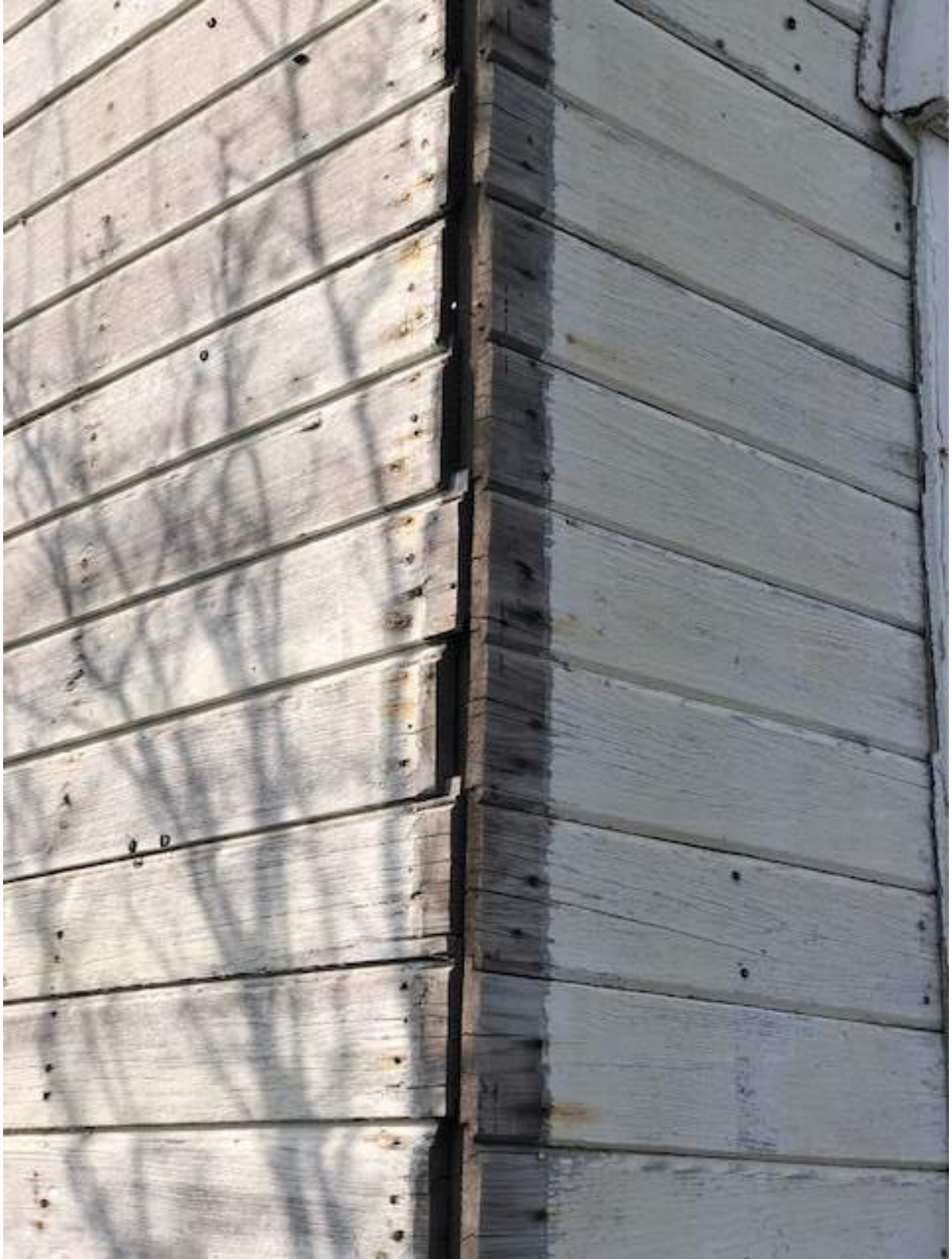
Missing trim at the left front corner.
