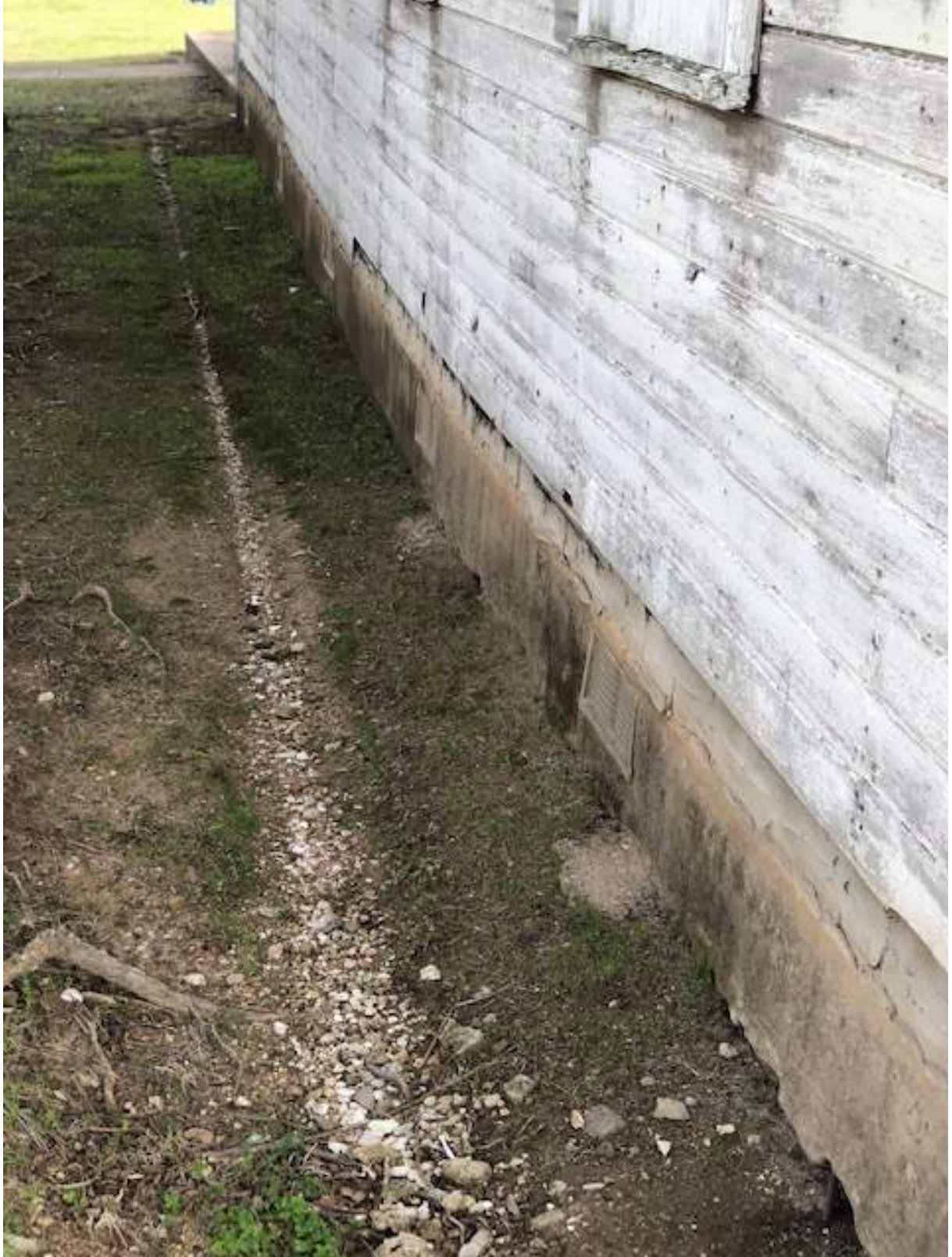
South side view shows drainage issues, current condition of siding.
