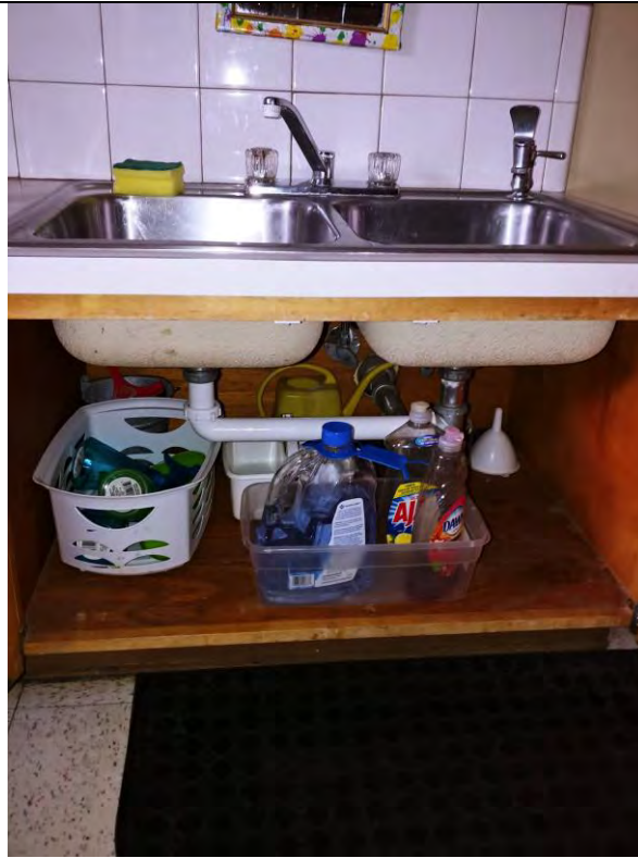
Photo 5: Sink located in the 4.5 to 5-year-old classroom.
