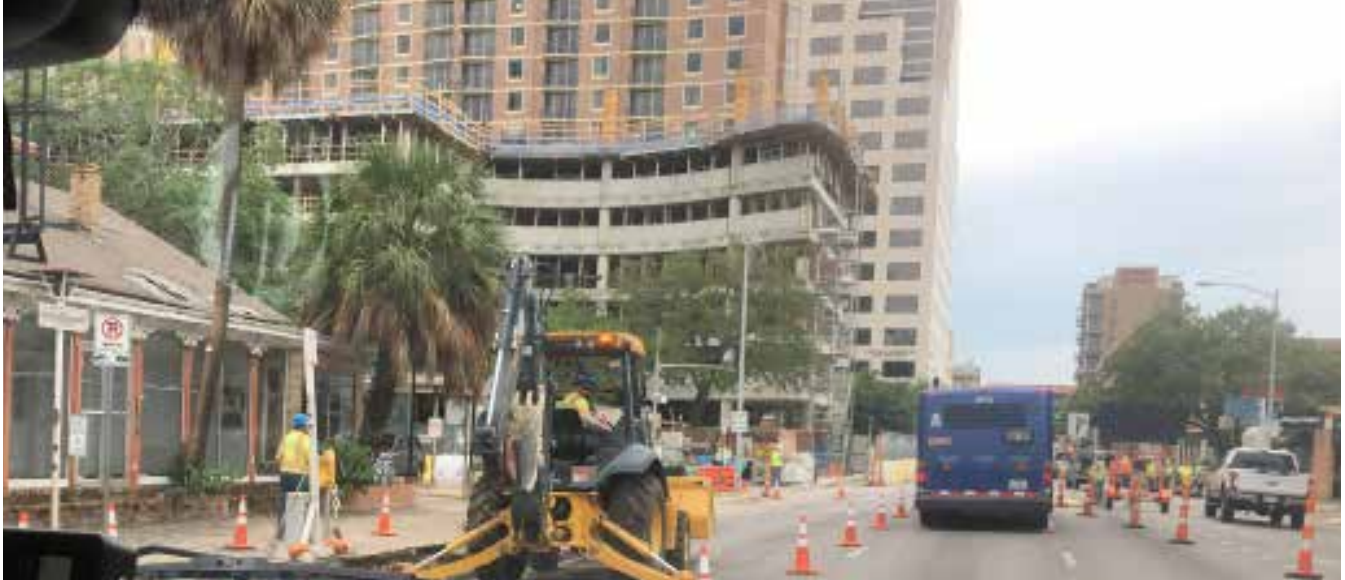
Source: OCA photo of Lavaca Street right of way conflict, June 2018
