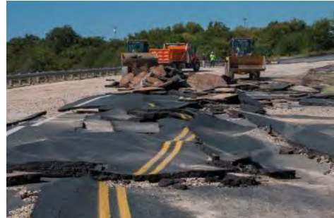
Roads, as well as other City-owned infrastructure, were damaged during the October 2013 floods.
