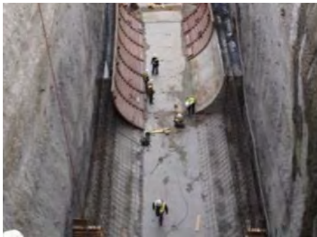
The Waller Creek Tunnel project, currently under construction, is being financed by a TIF.
