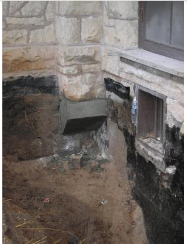
Cleanout assembly in French Drain
