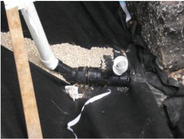
Cleanout Assembly in French drain
