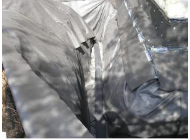
Perforated pipe in French drain
