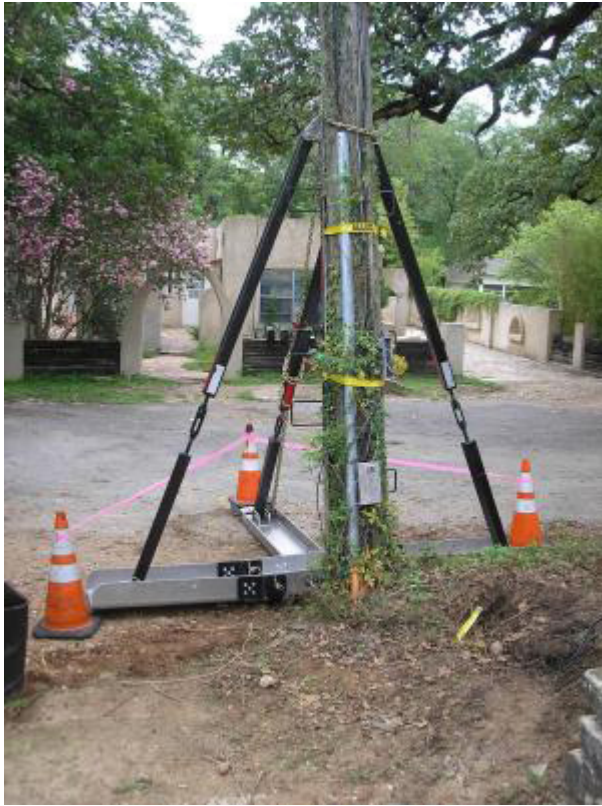
Utility Pole Support
