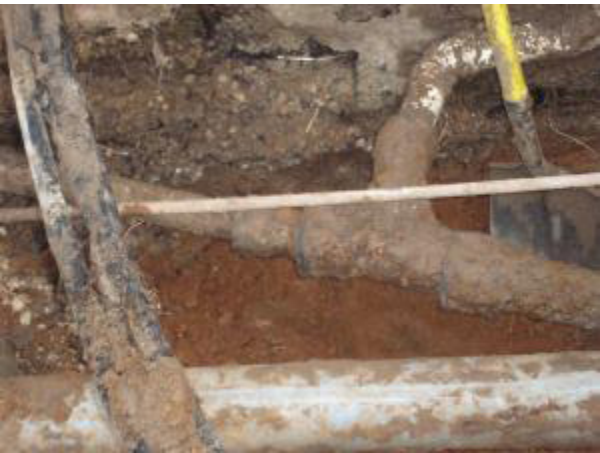
Leaking sewer pipe exposed
