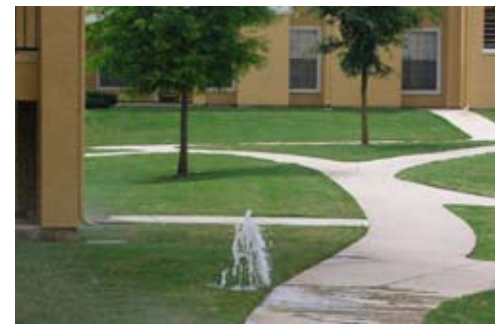
Broken spray head
