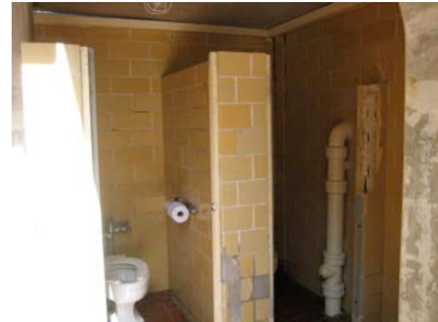
Aside from the deterioration, the preponderance of masonry toilet partitions gives the place a crowded feel. A rehabilitated Bathhouse should include more generous maneuvering clearances throughout.
