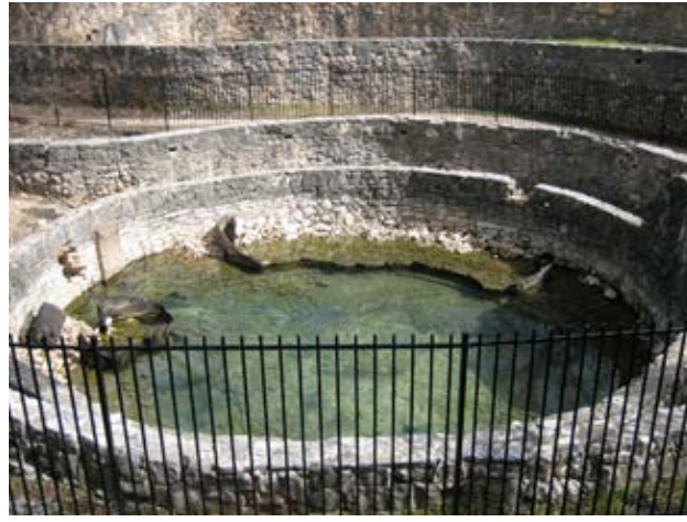
One short-term goal is to repair the walls of the spring vessel. In the same effort, add an operable sluice gate and remove sediment.
