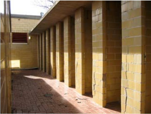
Aside from the masonry deterioration, some of the Women's Dressing area seems cramped and dank. Regular swimmers report that this area is rarely used.
