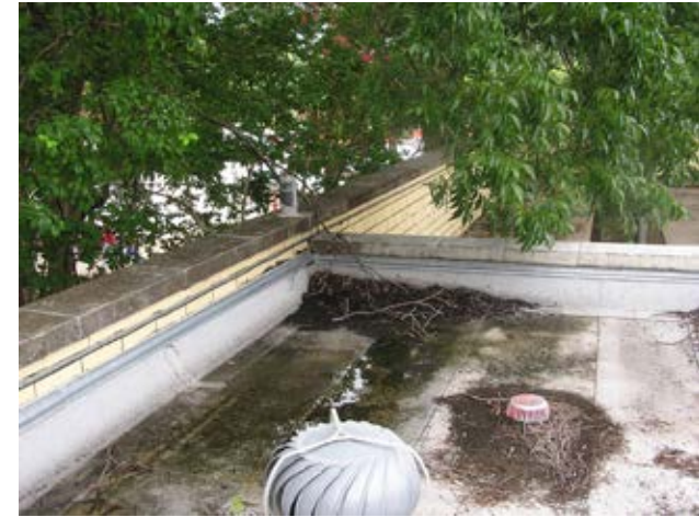
With a single area drain, and no overflow drain, a clog could lead to a catastrophic roof collapse.
