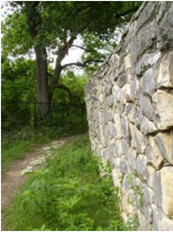
Some walls are leaning precipitously. Strategy for stabilization should account for historic preservation, long-term service and public safety.
