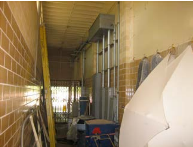
Electrical upgrades are installed unattractively, rendering this otherwise usable space good only for storage.
