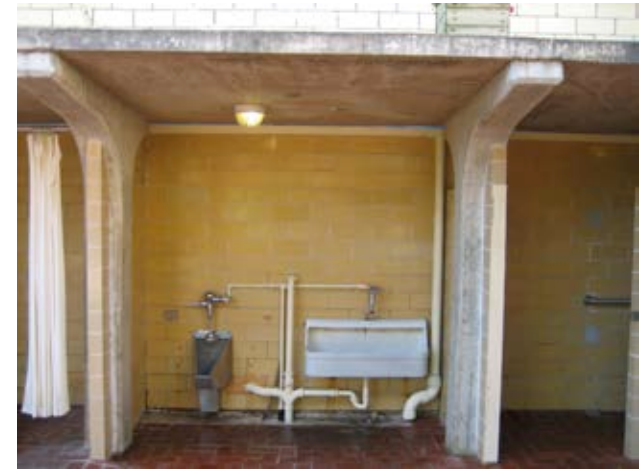
Plumbing fixtures vary in age and condition. Trough urinals (right) do not meet current code. None of the fixtures are low water-use fixtures.
