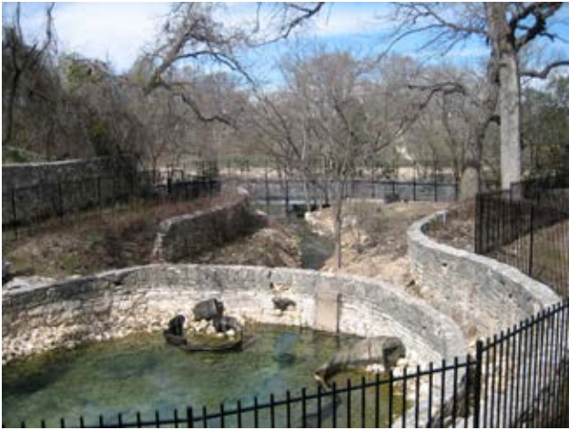
Sunken Garden in 2007. Some walls have collapsed, and the landscape is less organized. The fence is to protect the salamander habitat.
