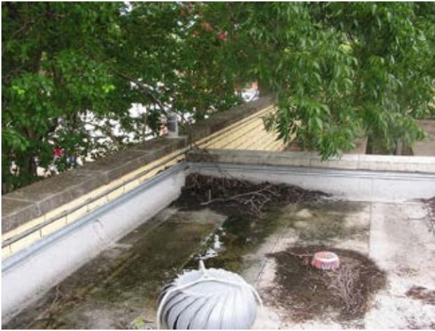
Certain roof areas are bordered by parapet walls that vary in height from a few inches to over three feet. These areas are drained by roof drains, but do not include overflow drainage provision.
