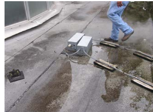
Most penetrations for roof top equipment electrical and refrigerant lines are voided and open.
