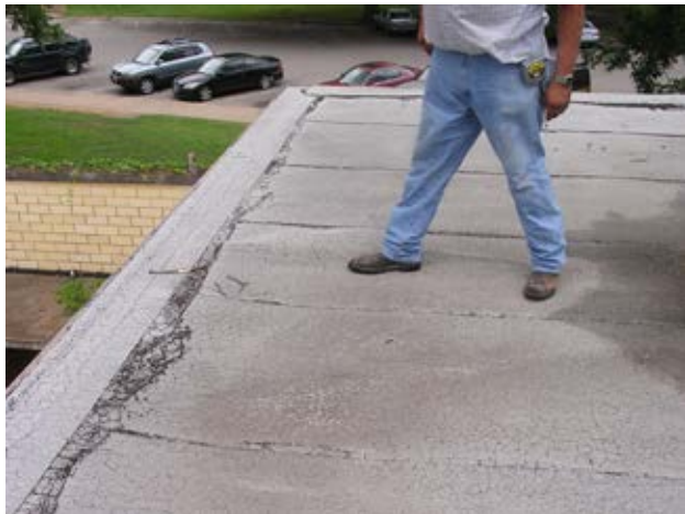
Many of the subordinate roofs are flat, and are surrounded by parapet walls. Because they are designed with a primary roof drain and no overflow drain, they do not meet today's code (above). Some of the roof membranes are pulling away from their substrates and puckering (below).
