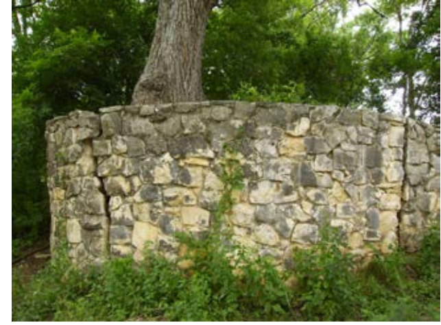
Repairing and stabilizing this crack will require the removal of the tree.
