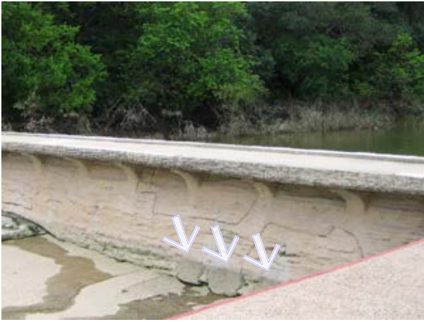
The upstream dam was built in the late 1920s with three openings in it for creek flow. These openings were closed during the 1975 construction of the bypass tunnel. One concept being considered is to install operable openings in the upstream dam.
