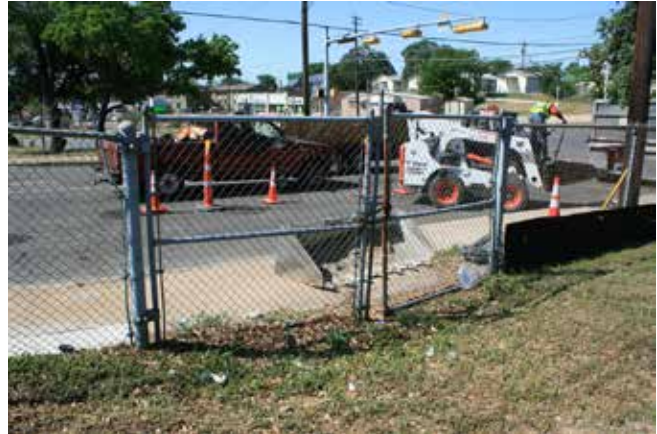
Figure 406. This chain link gate on East 12th Street previously allowed access to the house and garage. The fence and gate have since been updated. (John Milner Associates)
