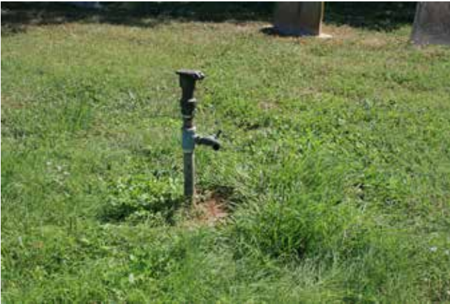
Figure 403. A steel pipe riser, part of Evergreen's underground irrigation system (John Milner Associates)
