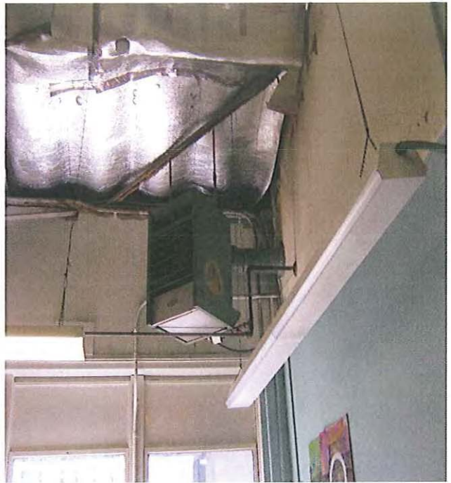
8. Ceiling/roof condition in Area B (5W).
