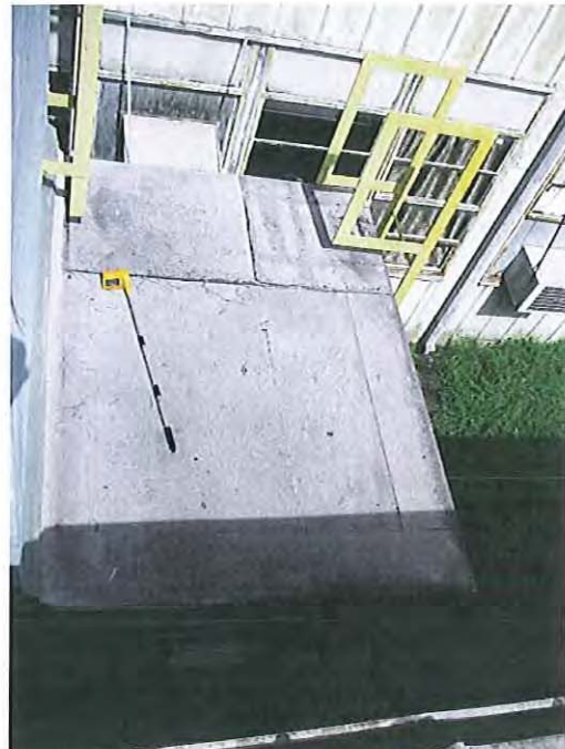
Photo A-6.1 Membrane aged, but serviceable.
