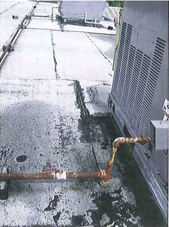
Photo A-3.3 Membrane decay at RTU.
