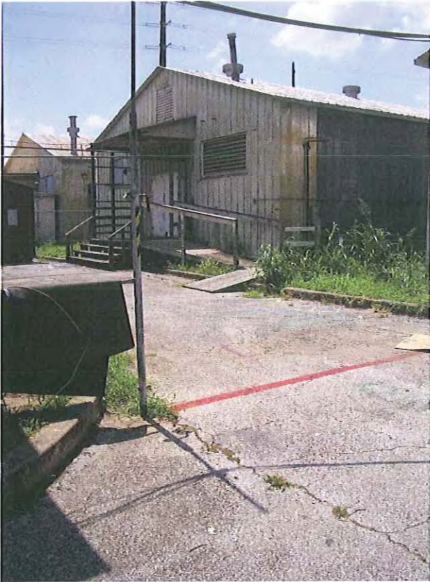
14. Exterior condition of Area C, emphasizing distinction between original and replacement wall panels.
