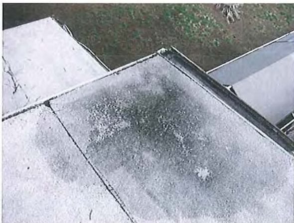
Photo A-2.3 Evidence of ponding in NW corner.
