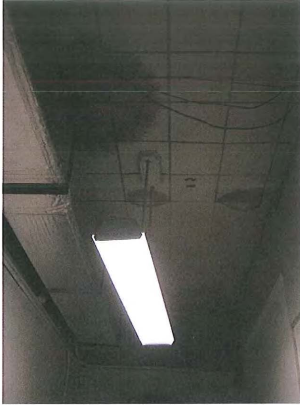
24. Evidence of roof leaks in Area E: typical corridor.
