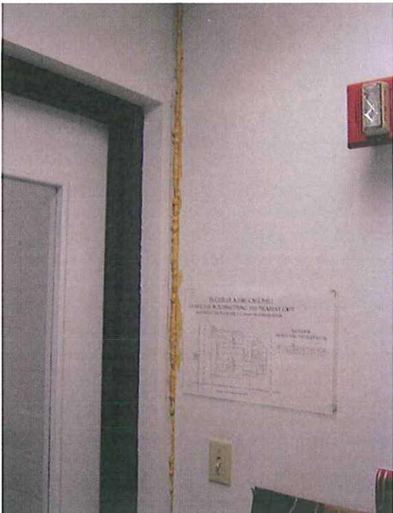
5. Conspicuous gap at staircase and 2 nd floor corridor west side of Area A
