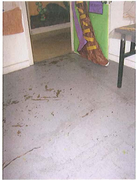
18. Evidence of past concrete repairs in Area D (8E).
