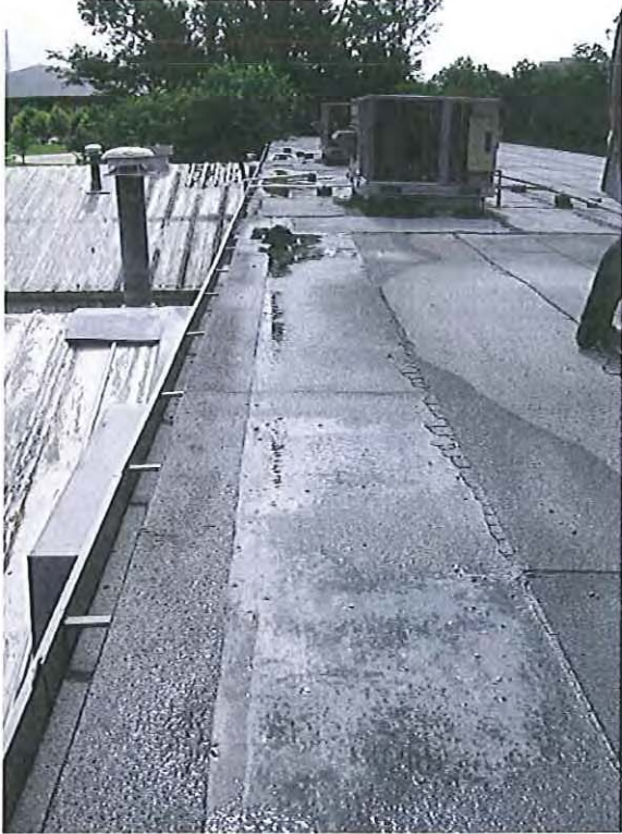
Photo A-3.2 Ponding along North edge.
