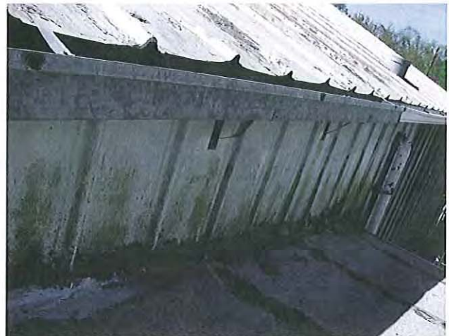
Photo B-1.4 Patchwork gutters – some sections are still serviceable; others are failed.
