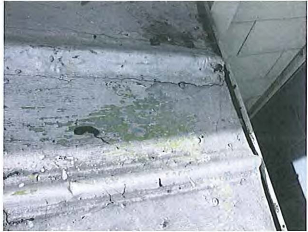
Photo D-1.2 Degradation at roof edge.
