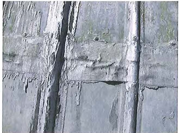
Photo C-1.2 Seal at lap joints not watertight.
