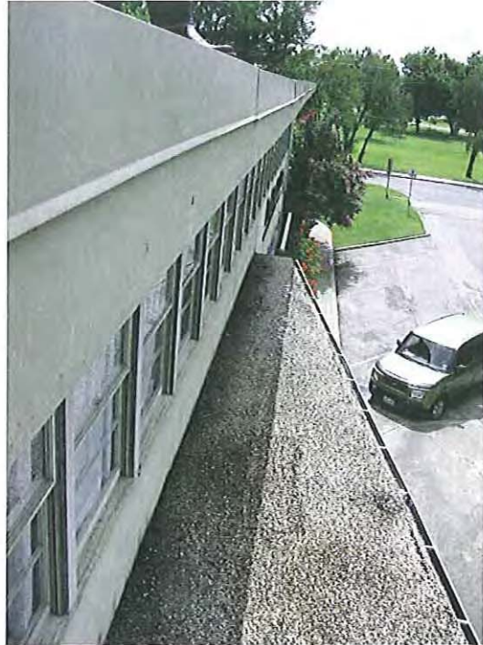
Photo A-4.2 East end of A4, gravel loss noted.
