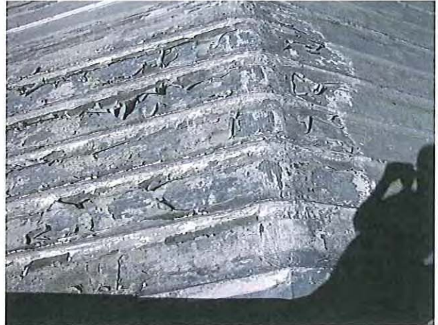
Photo B-1.2 Decayed roof patching.
