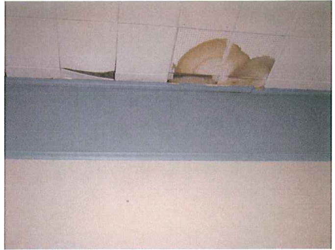
21. Evidence of roof leak in Area E (13N).
