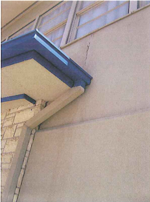
3. Failing plaster installation at Area A.
