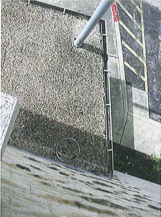
Photo A-4.1 West end of A4, gravel loss noted.
