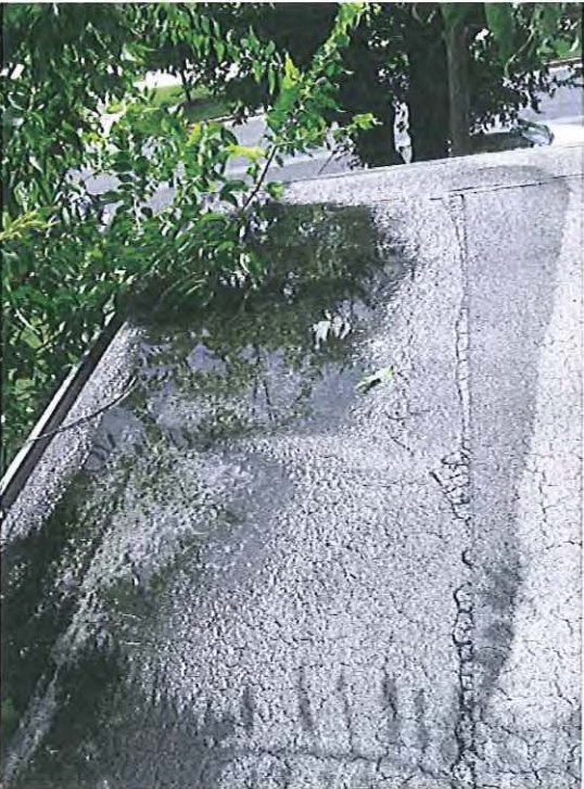
Photo A-3.4 Ponding at NE corner.
