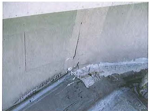
Photo C-1.4 Failing wall flashing.
