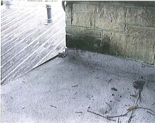
Photo A-1.1 Mold at wall flashing.
