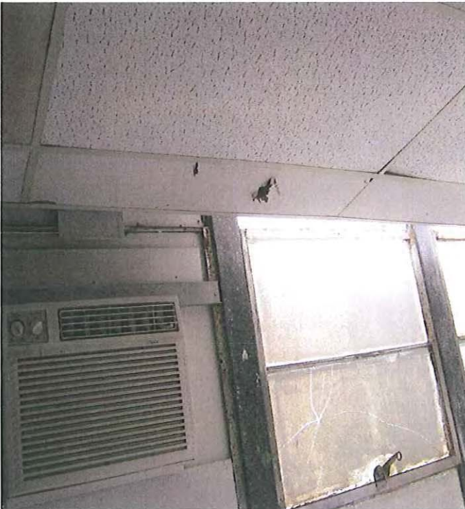
19. Evidence of vermin infestation and window failure in Area D (10E).
