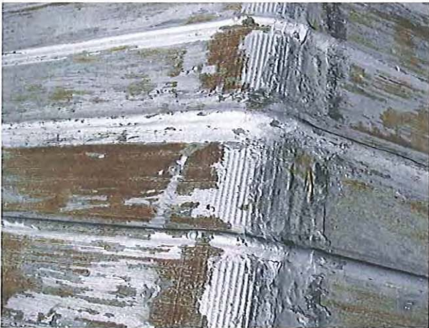
Photo B-1.3 Rusted panels, worn ridge sealing.
