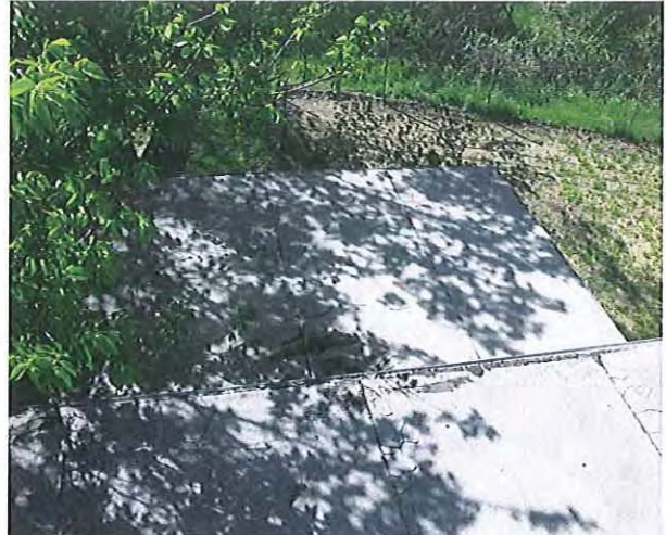
Photo A-1.2 Looking west. Damage at roof edge.
