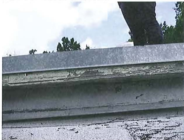
Photo A-2.1 Roof edge w/ weathered fascia.
