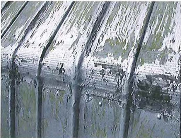
Photo C-1.3 Failing ridge patch.
