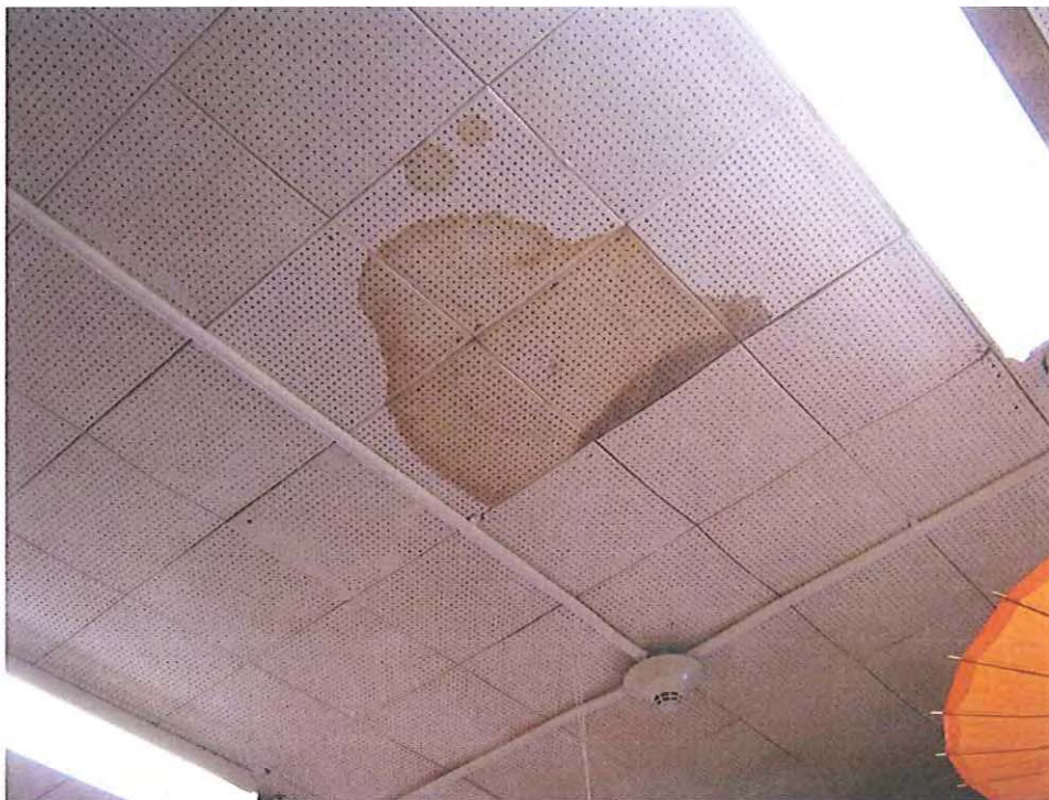
27. Evidence of roof leaks and pervasive water damage in Area E.
