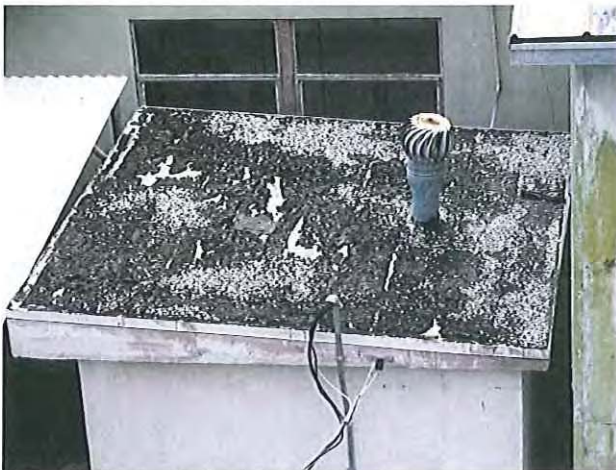
Photo D-2.1 Failed Membrane.
