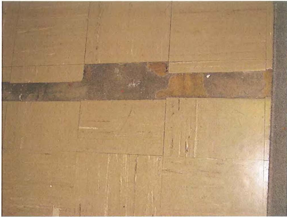
28. Typical tile conditions throughout Area E
