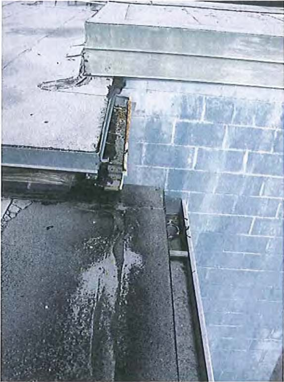
Photo A-3.1 NW corner w/ evidence of ponding.
