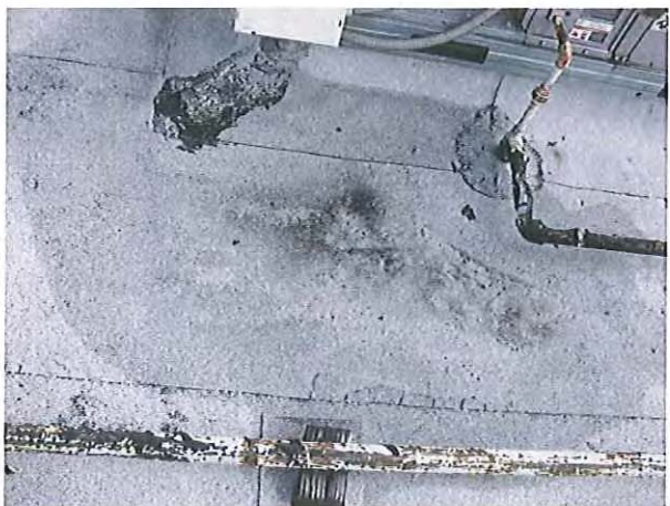
Photo A-2.4 Evidence of ponding near RTU.
