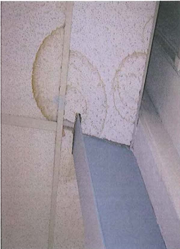
9. Evidence of roof membrane failure in Area B (4W).
