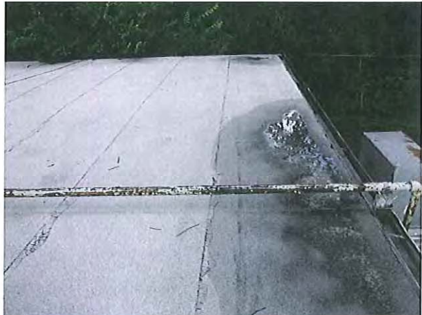
Photo A-2.2 Looking west, ponding at roof edge
