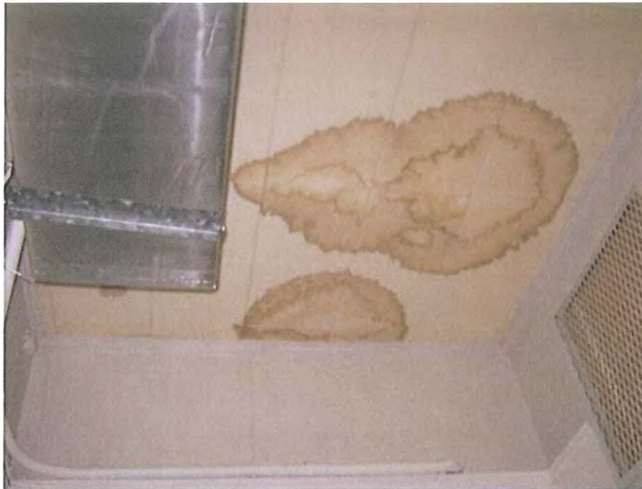
26. Evidence of roof leaks in Area E.
