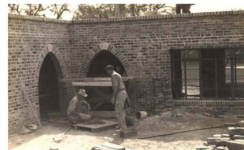
C Caretakers and Shelter House under construction in 1941 at Parque Zaragoza, now referred to as the Bath House (AHC, PICA 24236, 1941)
