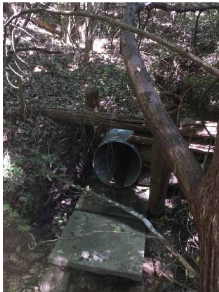
Figure 7: Culvert near Discovery Center property line northeast side of the property that drains north toward the road.
