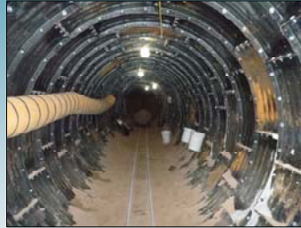
Tunneling operation to install a new 72-inch RCP under the CapMetro Redline
