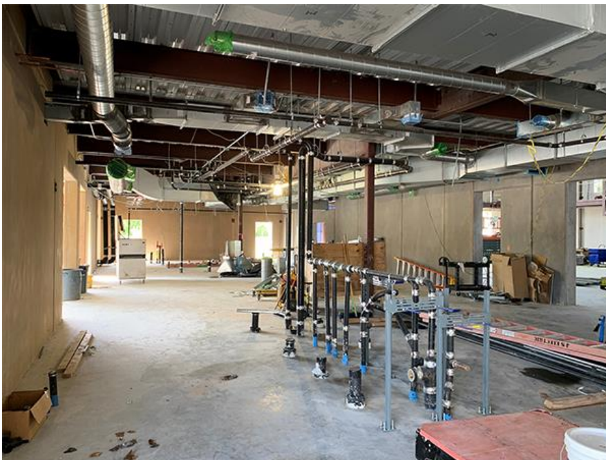
Interior shot of south building. Overhead mechanical, electrical, and plumbing installed
