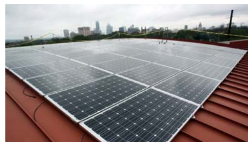
Carver Library Solar PV
