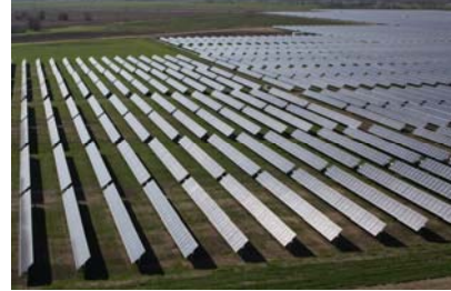
Webberville Solar Farm
