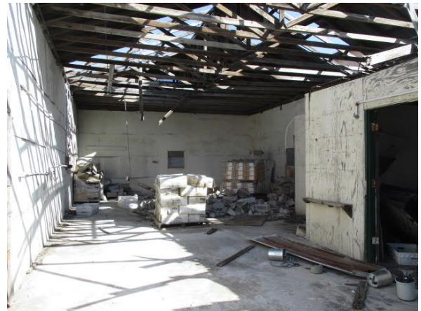
Photo 18 General interior view of the on-site building adjoining the 6915 Ryan Drive building
