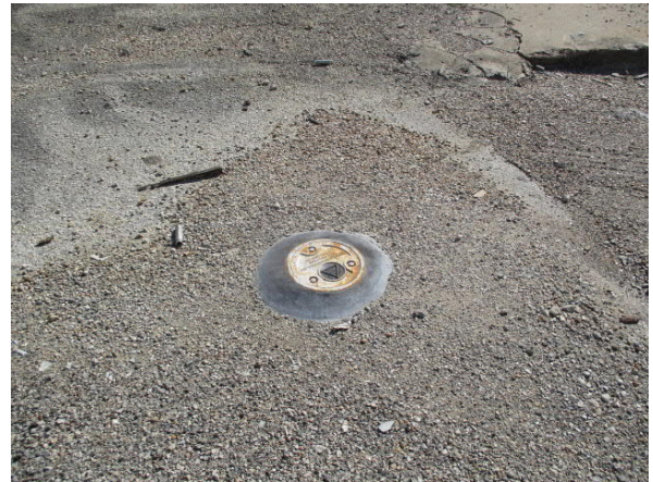
Photo 22 General view of an on-site monitoring well
