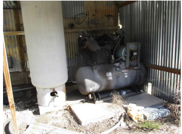
Photo 2 General view of the two on-site air compressors
