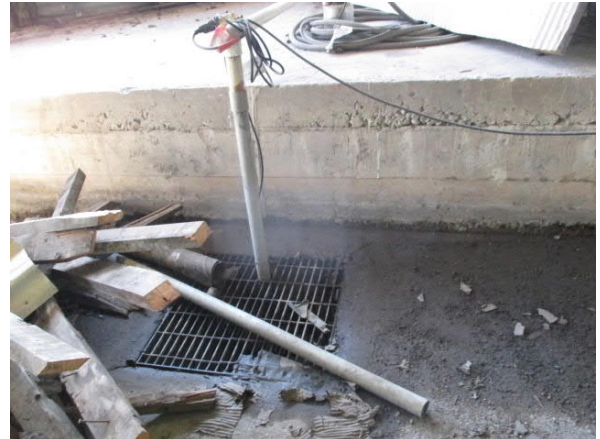
Photo 8 General view of the sump observed within the on-site 920 Justin Lane building
