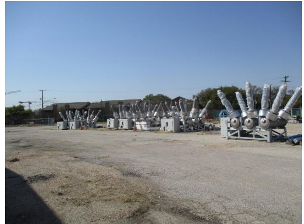
Photo 26 General view of the City of Austin's Austin Energy division equipment storage
