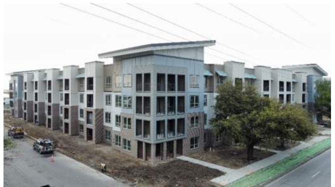
Westmoreland Station (248-unit multi-family development in Dallas, Texas at 2700 S Westmoreland Rd.) construction progress photo dated 3/22/2023.
