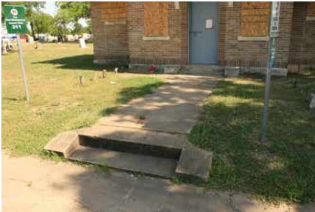
Figure 239. A concrete sidewalk and short set of steps lead to the restroom/gatehouse. (John Milner Associates)
