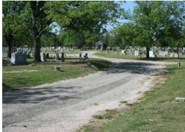
Figure 237. The curving cemetery drives are deteriorated at the edges. (John Milner Associates)
