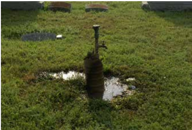
Figure 262. Dripping faucet with ponding (McDoux Preservation)
