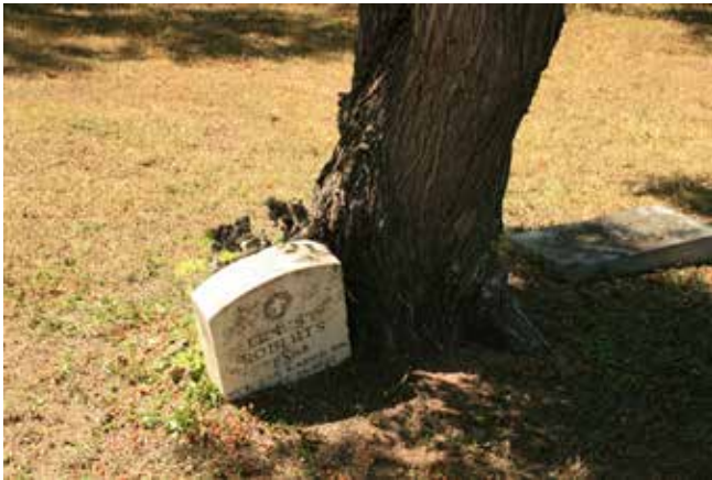
Figure 306. Tree roots causing damage to adjacent markers (John Milner Associates)
