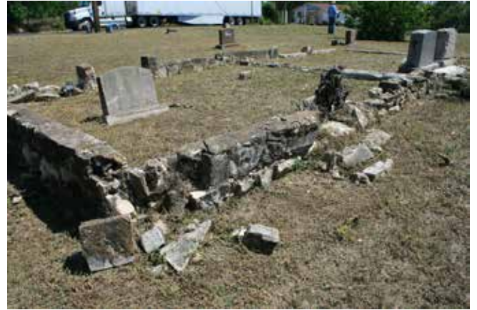
Figure 333. A severely damaged plot enclosure (John Milner Associates)
