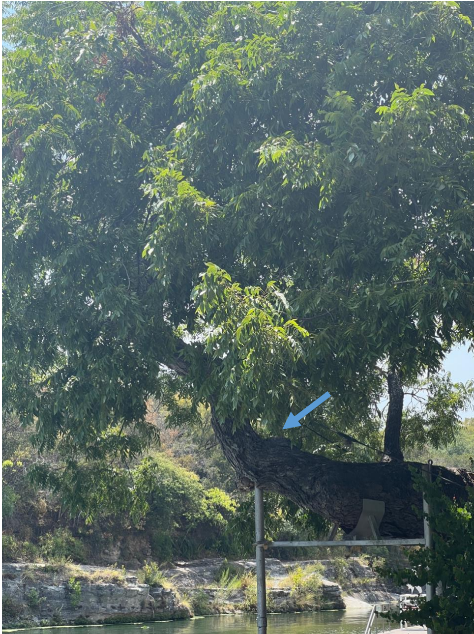
5: second support, defect location, and size of part of concern
