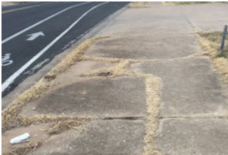
Severe cracking creates uneven and hazardous walking surfaces
