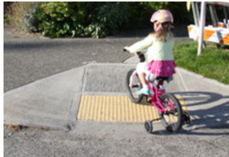
A sidewalk retrofitted with a curb ramp and a tactile warning strip
