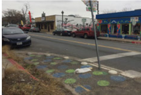
Easy-to-install materials such as paint, turtle bumps, and flex posts may be used to create curb extensions
