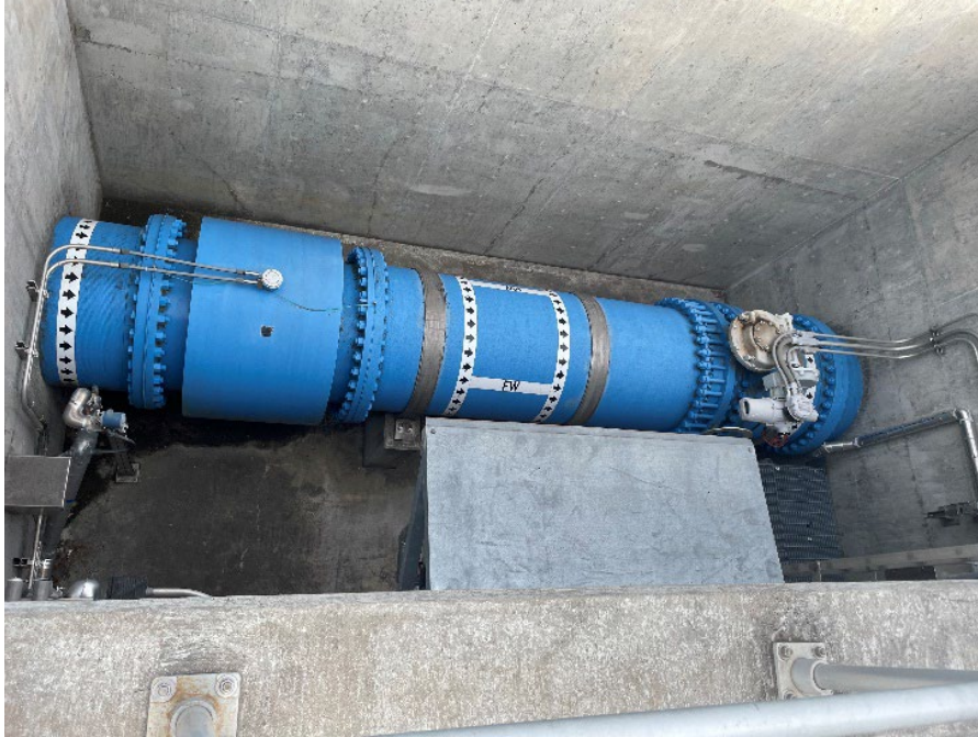
Figure 3-2 Handcox WTP Finished Water
