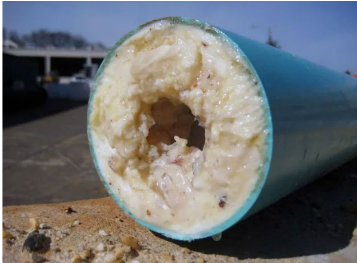
Fuente de la imagen: Opinion: 'Fatbergs' of Holiday Grease Dangerously Clog California Sewage Systems
