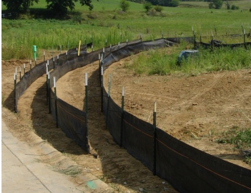
Silt fencing is placed at the “limits of construction” to catch sediment before it runs offsite and into a creek. The bare soil becomes sediment when it’s mobilized by stormwater runoff.
